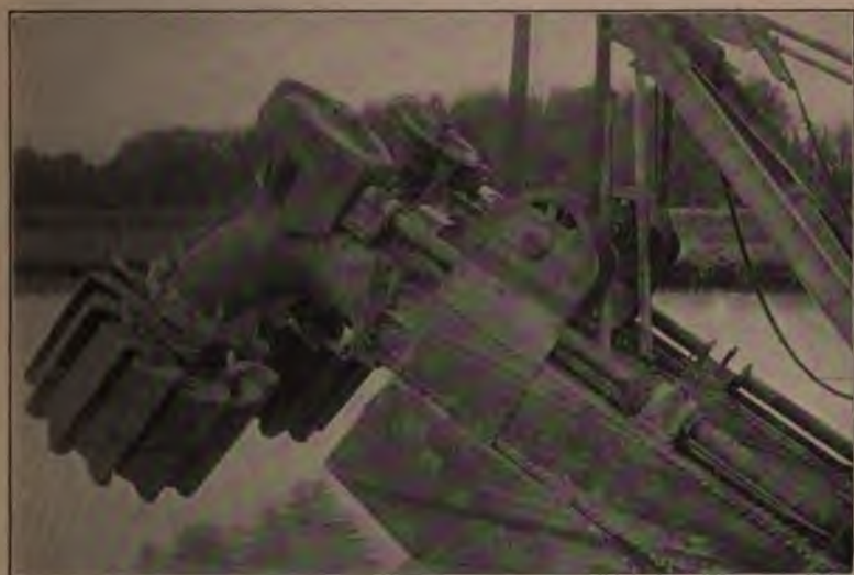
Cutter Heads and Suction Pipes of Hydraulic Dredge Operating on New York State Barge Canal.
